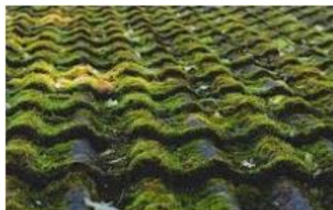
Figure 8: Moss growing on a rooftop
